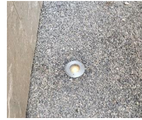
Figure 15: Exterior light on at 12:00 noon
