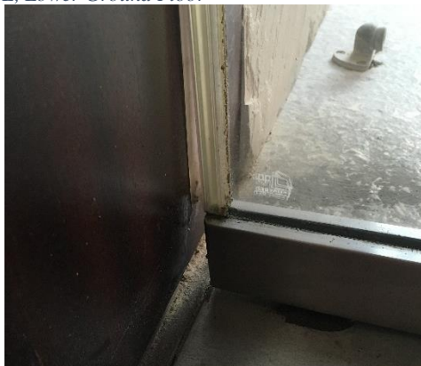
Figure 14: Large Door gap in the Majlis
