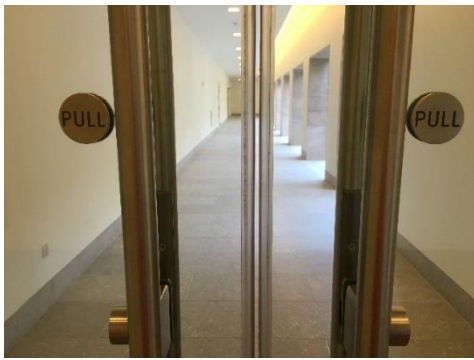
Figure 13: Open gap between doors in Segment E, Lower Ground Floor
