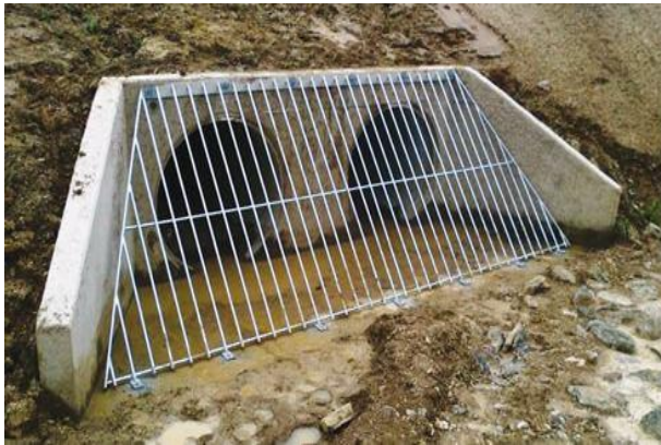
Figure 17 - Custom culvert grate
